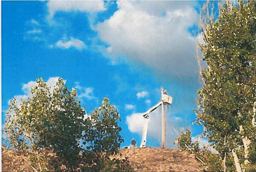
Crews installing a new power pole on Beaver Creek. Photo by Marcy Stamper
